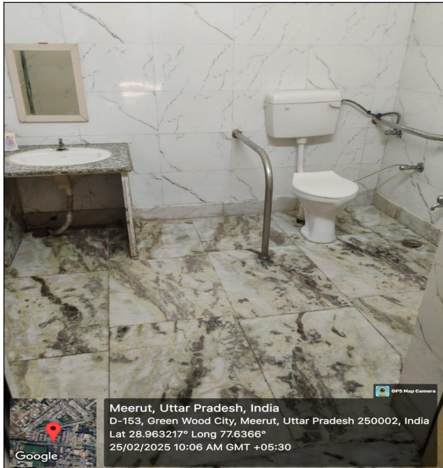
WASHROOM IN LALA HARDAYAL BHAWAN HOSTEL
