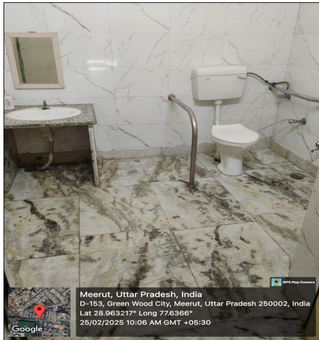
WASHROOM IN LALA HARDAYAL BHAWAN HOSTEL
